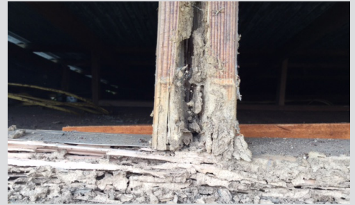
Extensive termite damage in the apartment
