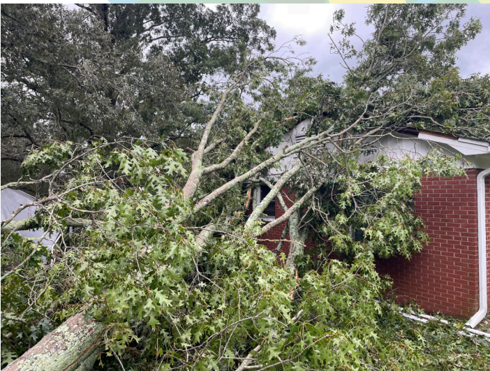
A tree fell on our home during Hurricane Helene.
