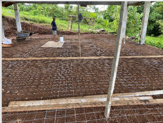
The mesh wire has been placed for the floor, and we are waiting for the cement to be poured.
